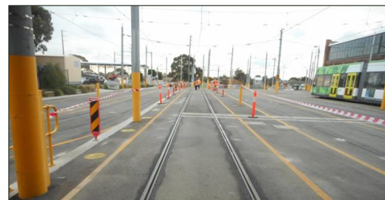
Figure 6. New Preston Depot Test Site for Braking Trials
