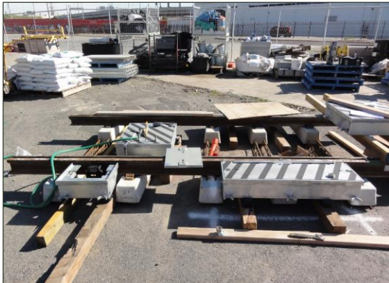
Figure 11. Pre-installation TOR equipment Mock-up Site
