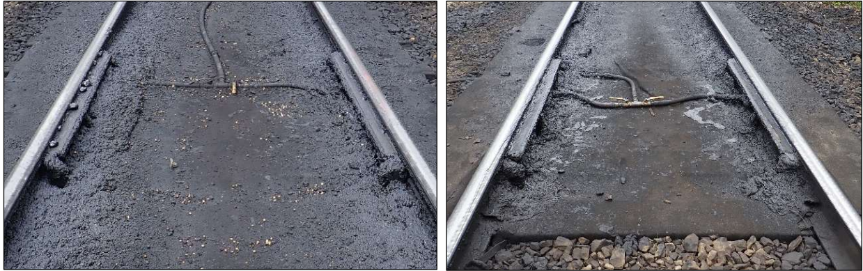
FIGURE 11: Common examples of port clogging recorded with tradition petroleum grease application.
