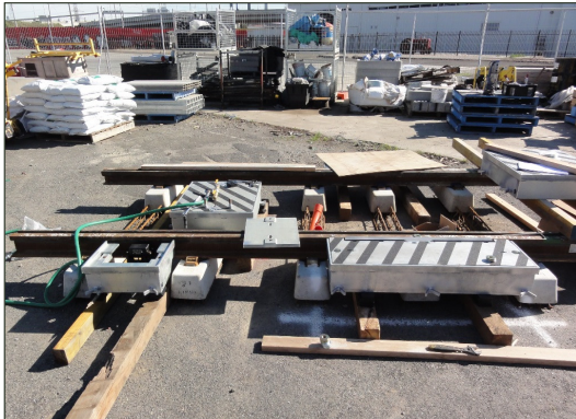
Figure 11. Pre-installation TOR equipment Mock-up Site
