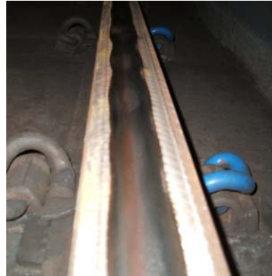
Figure 2 Typical low rail corrugations between CTA and T4
